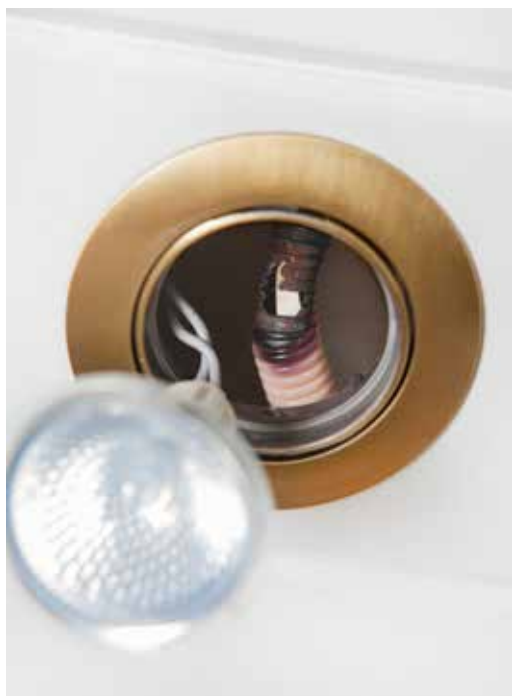
Feilinstallert downlights, her kan det fort gå galt.
